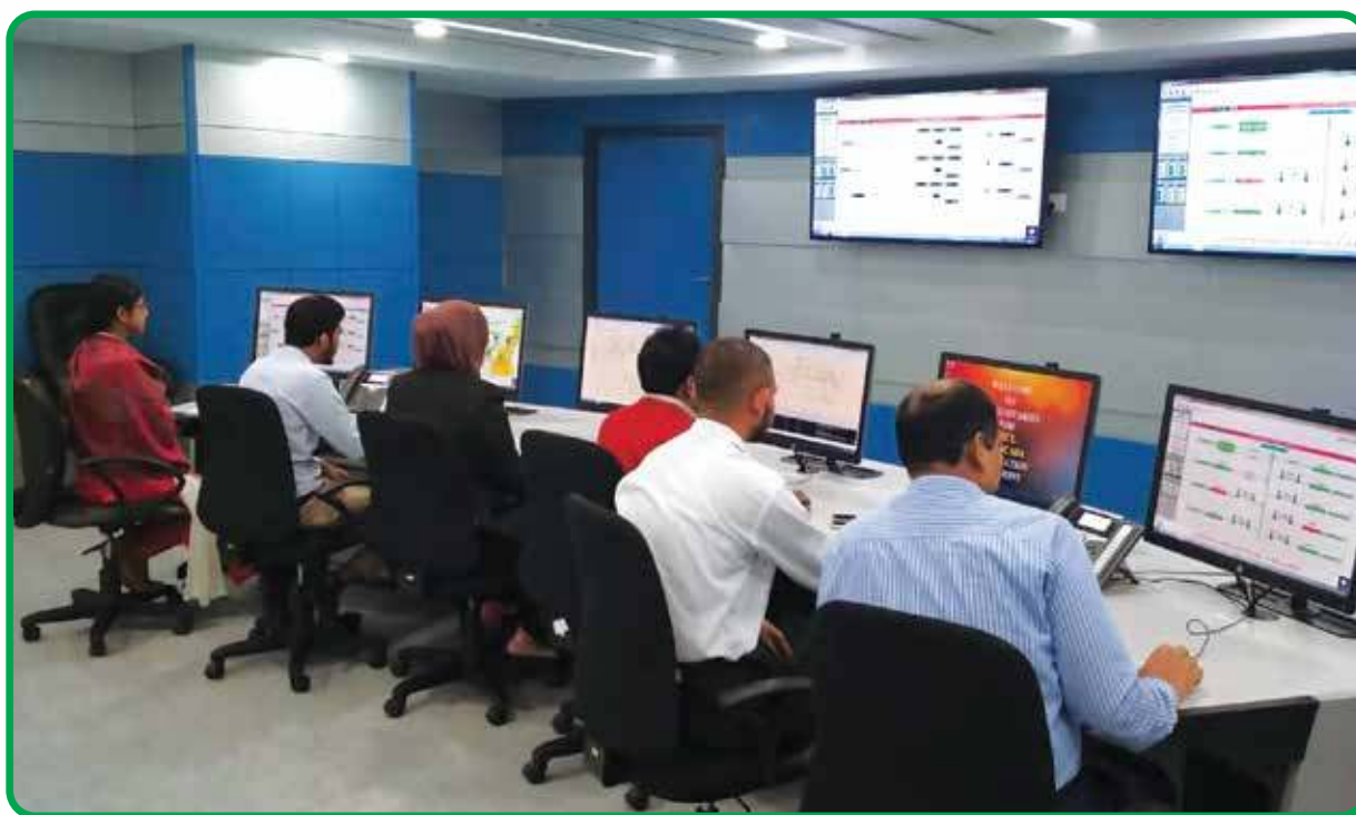
SCADA Master Control Centre at GTCL Head office building, Agargaon, Dhaka
