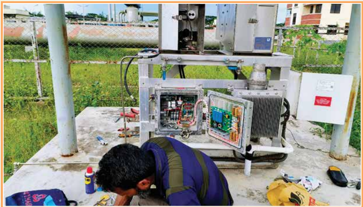
Cathodic Protection systems maintenance works for corrosion mitigation of Gas transmission pipeline
