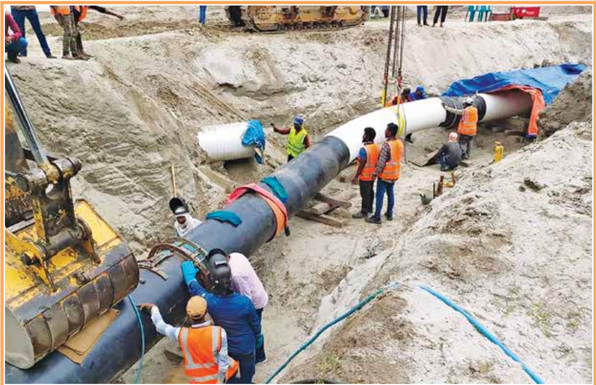
Replacement works of 30" dia gas pipeline from Elenga to east side of Bangabandhu bridge under SASEC-2
