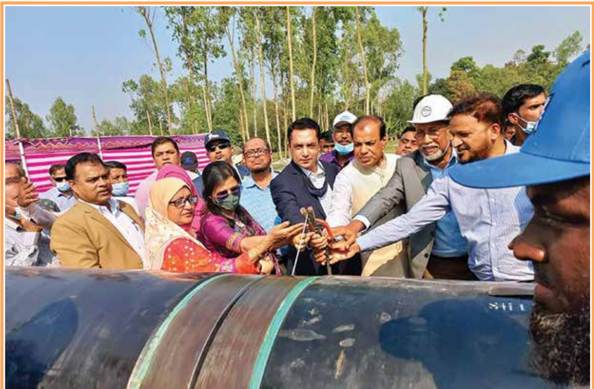
Inauguration of welding works of Section-C under Bogura-Rangpur-Sayedpur Gas Transmission Pipeline Project
