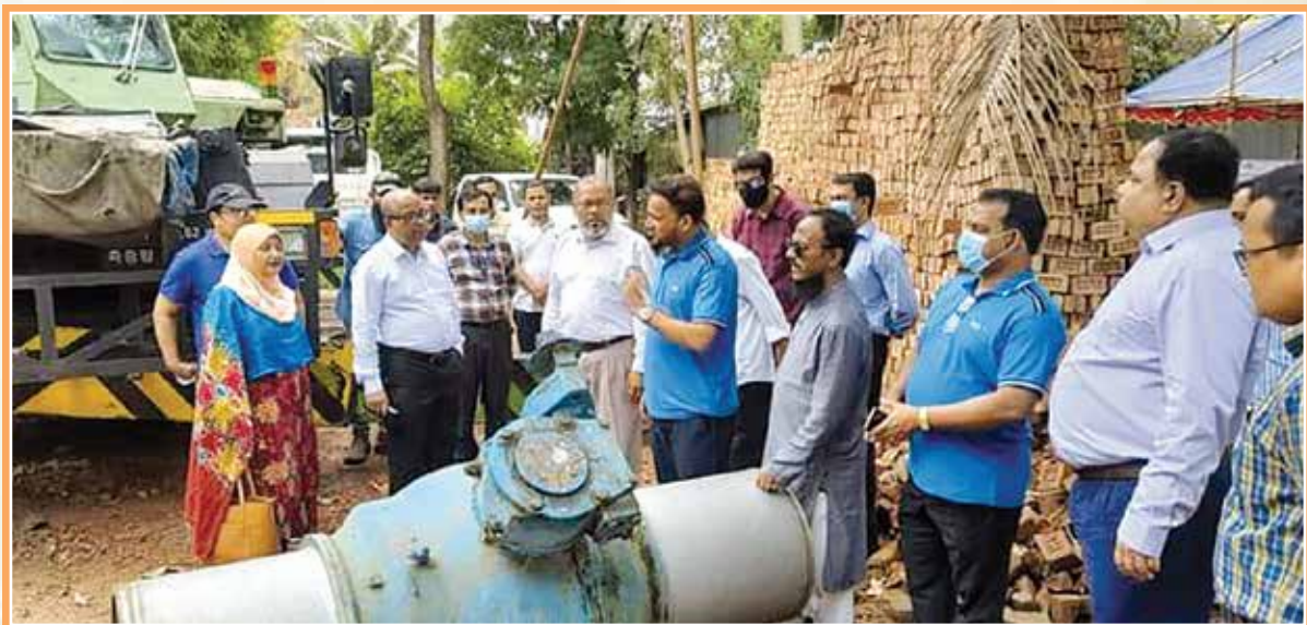
Replacement works of 20" dia Valves at Kodda and Panshail Valve Station under Dhanua-Savar Gas Transmission Pipeline were visited by Honorable Chairman, Petrobangla along with MD, TGTDC & MD, GTCL
