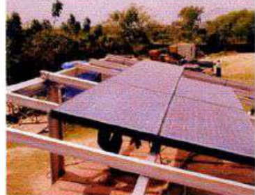
Solar Panel Array
