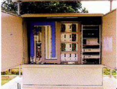
Remote Terminal Unit
